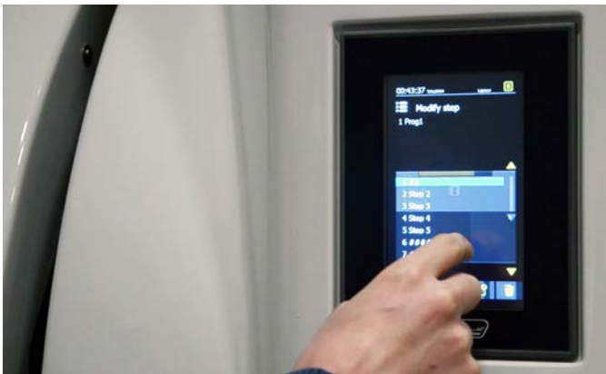
Picture: Siemens microprocessor control system
